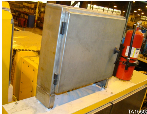
Air box mounted on top of the low voltage control cabinet
